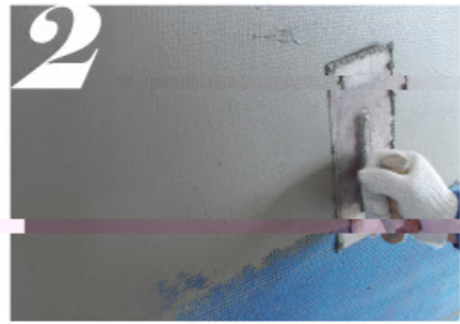
2 涂刷抗裂砂浆复合耐碱玻纤布 Coat with anti-crack mortar composite alkali-resistant mesh
